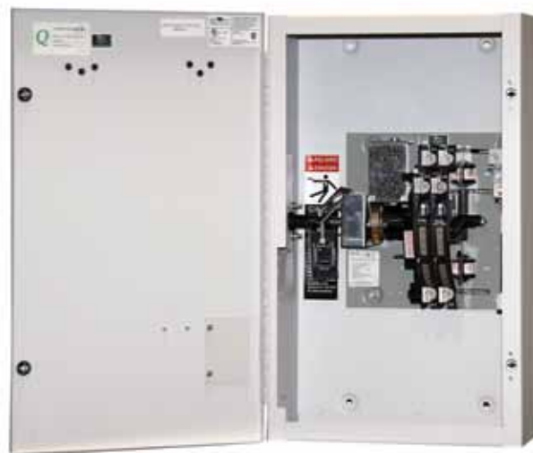
185 Manual Transfer Switch Door Open
